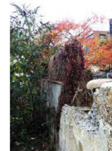
Wall Fence in disrepair
